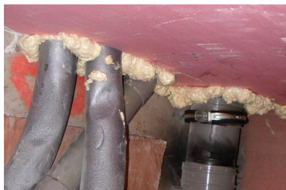
Incorrect use of PU 'foam' in a penetration seal
