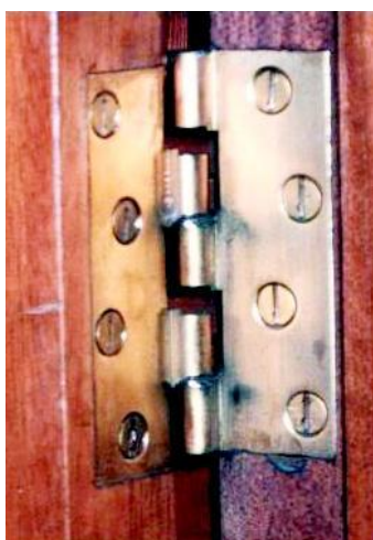
Worn hinges allow the door to drop
