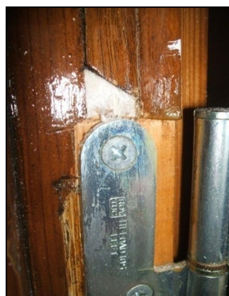
Replacement hinge is unsuitable and badly fitted to door
