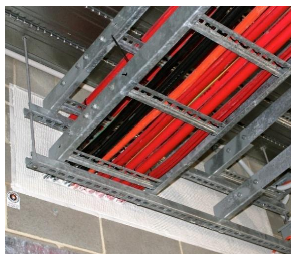
Correctly installed cable penetrations
