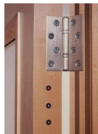
Intumescent seal in door frame
