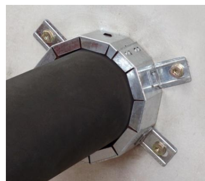
Caption - correctly installed pipe penetration
