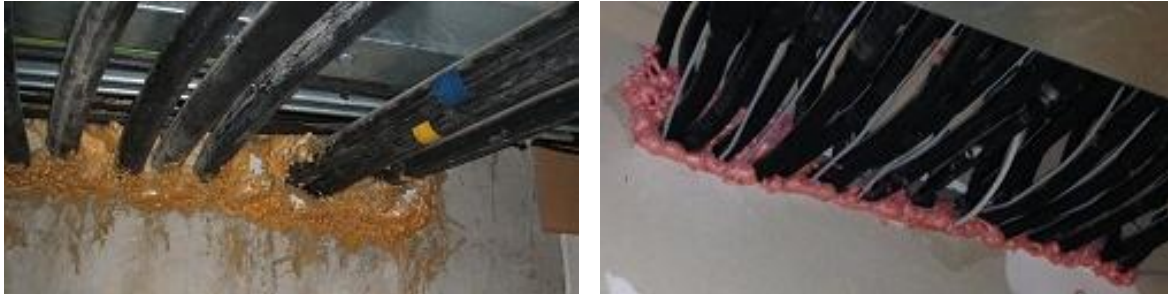
Above: Examples of Firestopping seals that are unlikely to be supported by test and certification.
