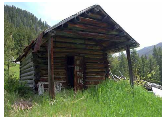
Opposite: Tiedowns are at the south end. Above: Mountain bikers can ride 3 miles to this old cabin above Smith Creek Bridge.
